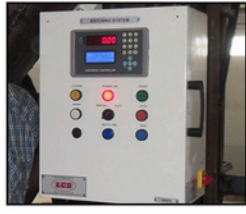
Batch Weighing System
